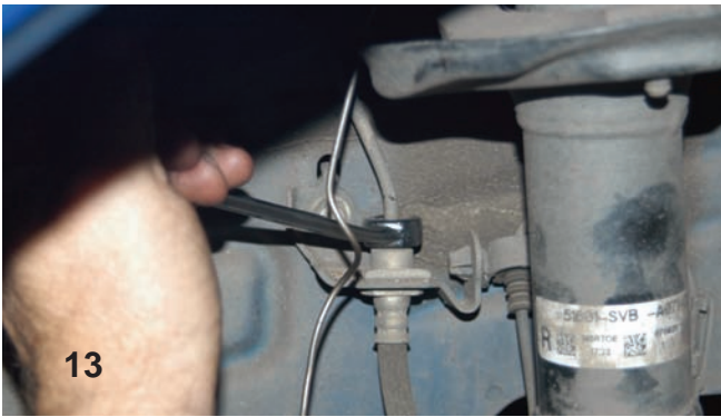
13 Using a line wrench, the hard line was disconnected from the original flex line.
