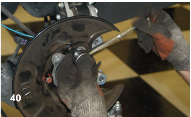
Using a socket wrench and the correct size socket, the small bolts that connect the dust shield to the strut assembly were removed.
