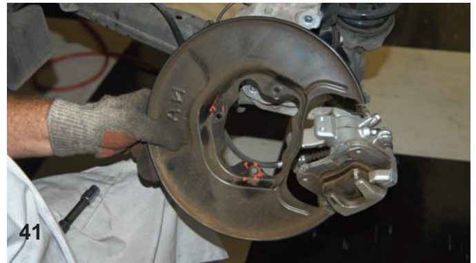
The dust shield was removed from the strut assembly and it will not be reused.
