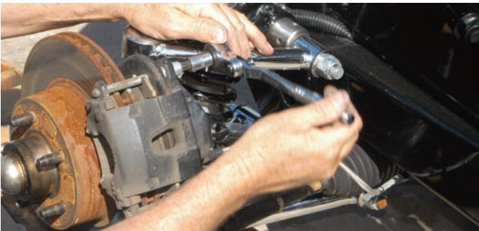
The GM calipers were removed by disconnecting the two special Allen head bolts as seen here. There is one on each side of the single piston caliper.
