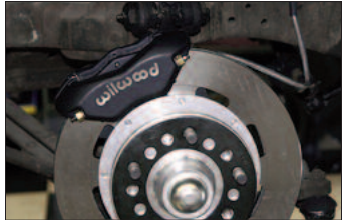
Sequence 22: Connect one end of the flexline to the previously installed caliper fitting. Route line along a similar path as the OEM hose.
