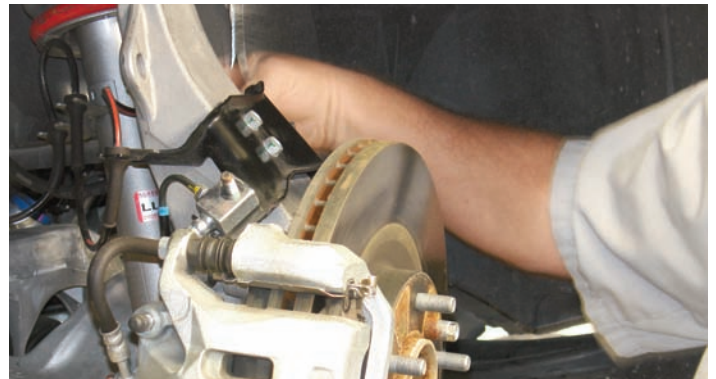
You can't see it from here but Tony is removing the caliper brake line with a line wrench. This car has a very unusual front brake line engineering.
